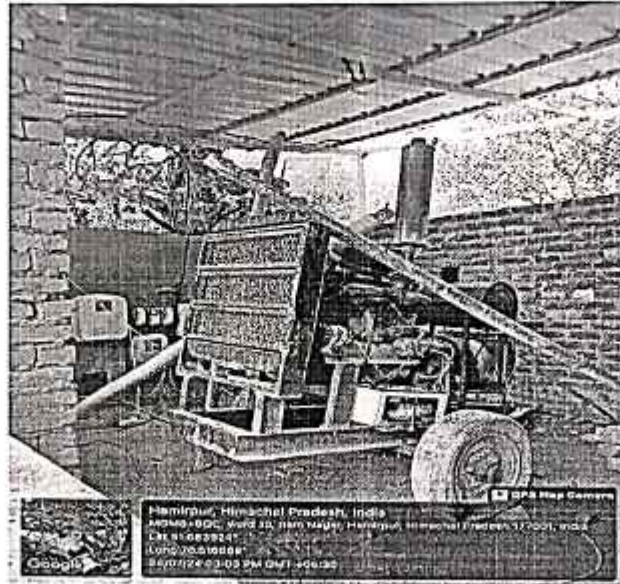
Picture of Generator available at Gautam College of Pharmacy
